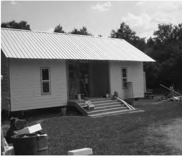
FIGURE 12. 20K House IX. Built by “outreach” students at the Auburn University Rural Studio under the direction of Andrew Freear (studio director) and Danny Wicke (20K instructor), 2009–2010. Photo by author, summer 2010.
