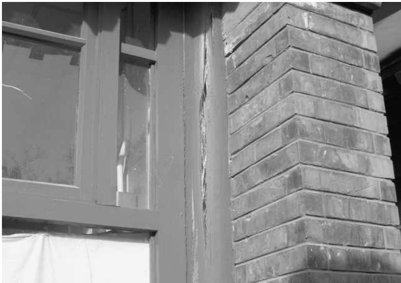
FIGURE 18. A cracked exterior column at a renewed courtyard house on Qingfeng Hutong.
