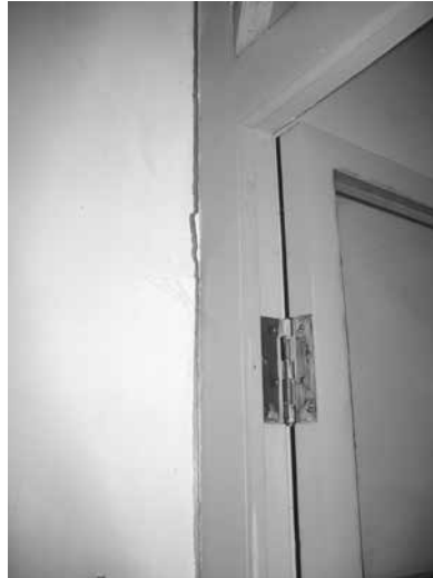
FIGURE 16. (LEFT) Crack at the interior junction between a column and a wall in a renewed courtyard house on Qingfeng Hutong. FIGURE 17. (RIGHT) Crack at the interior junction between a doorframe and a wall in a renewed courtyard house on Qingfeng Hutong.
