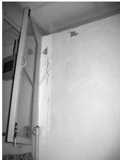
FIGURE 19. (LEFT) Unsupported by the doorframe, a beam's weight rests on a window at a renewed courtyard house on Qingfeng Hutong. FIGURE 20. (RIGHT) Wall cracks and an unhinged window frame at a renewed courtyard house on Qingfeng Hutong.
