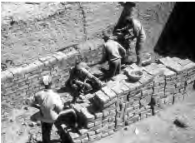
FIGURE 9. A coordinated arrangement of laborers who pass materials onto an apprentice setting brick courses for a new wall.
