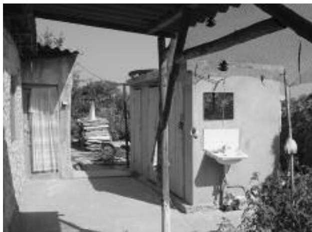
FIGURE 6. In the case of small, existing houses, where there was not enough space inside for a bathroom, it was built separately, in the courtyard. Here an old structure encloses toilets and a shower at Vasile Egor's house, 2 Mai, 2006.
